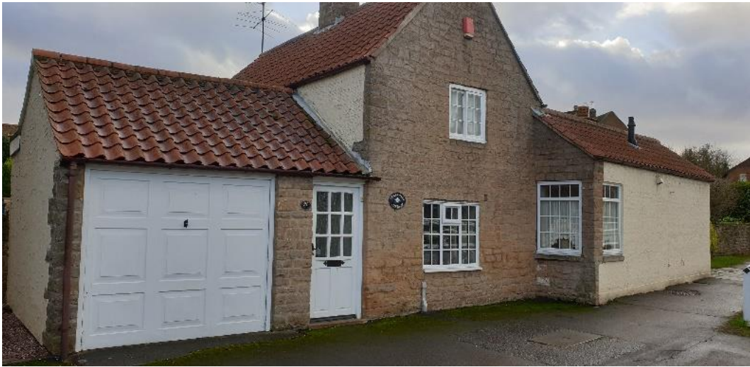
Photo 59 – Painting over stonework should be avoided
